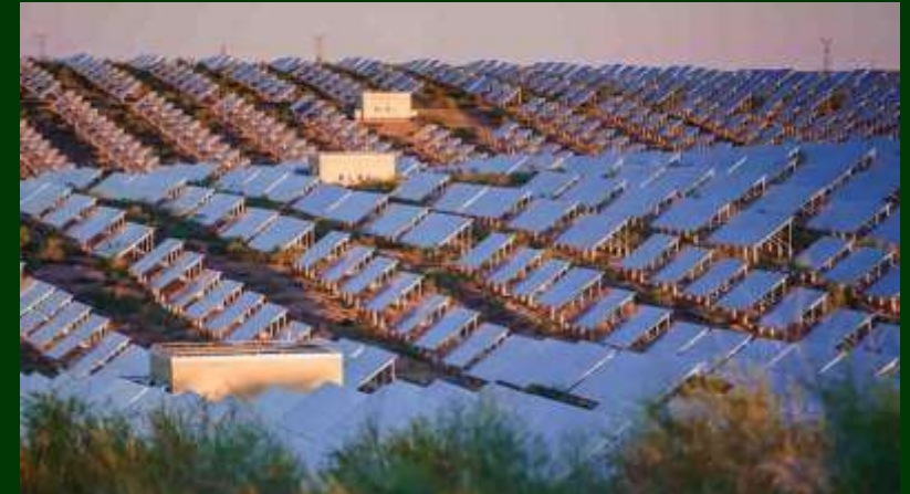
China's First Sand-Solar Hybrid Power Station 310MW | Kubuqi, Inner Mongolia, China
